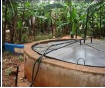
Bio gas plant
